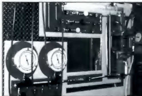
The Gas Station's state of the art blending panel can supply, enriched air nitrox, heliox, trimix, oxygen, argon to your specifications.
